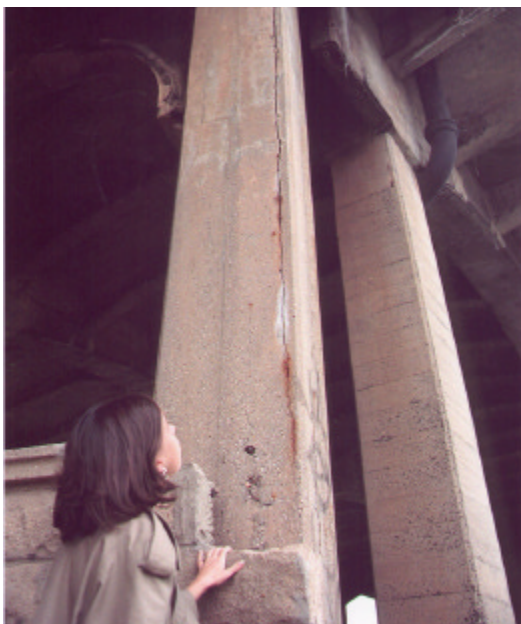
Tri-State Transportation Campaign executive director Janine Bauer inspects crumbling Route 1&9 viaduct during 1996 "fix-it-first" press conference
